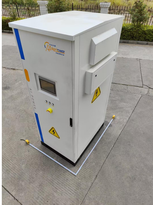
Photo 1 电池组正面 Front view of battery
